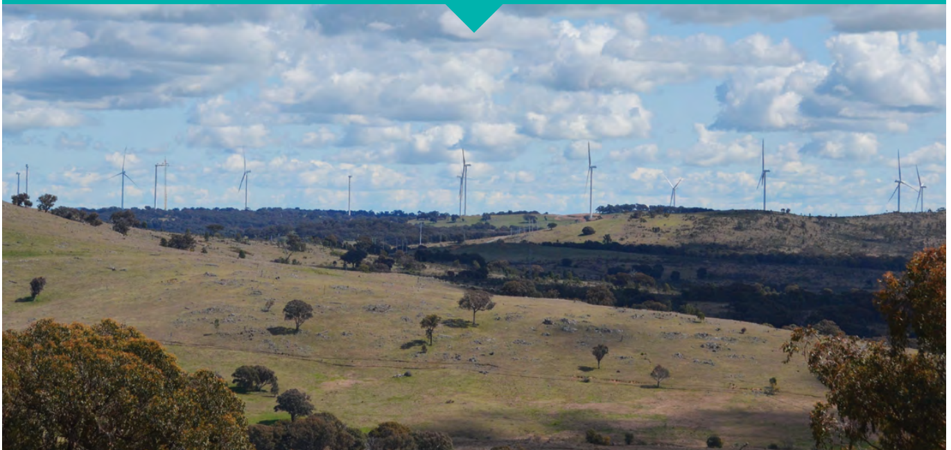
Bango Wind Farm western cluster where lifting of components is nearing completion.
