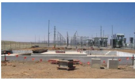
Transformer foundation (foreground) and electrical substation and switchgear infrastructure (background)
