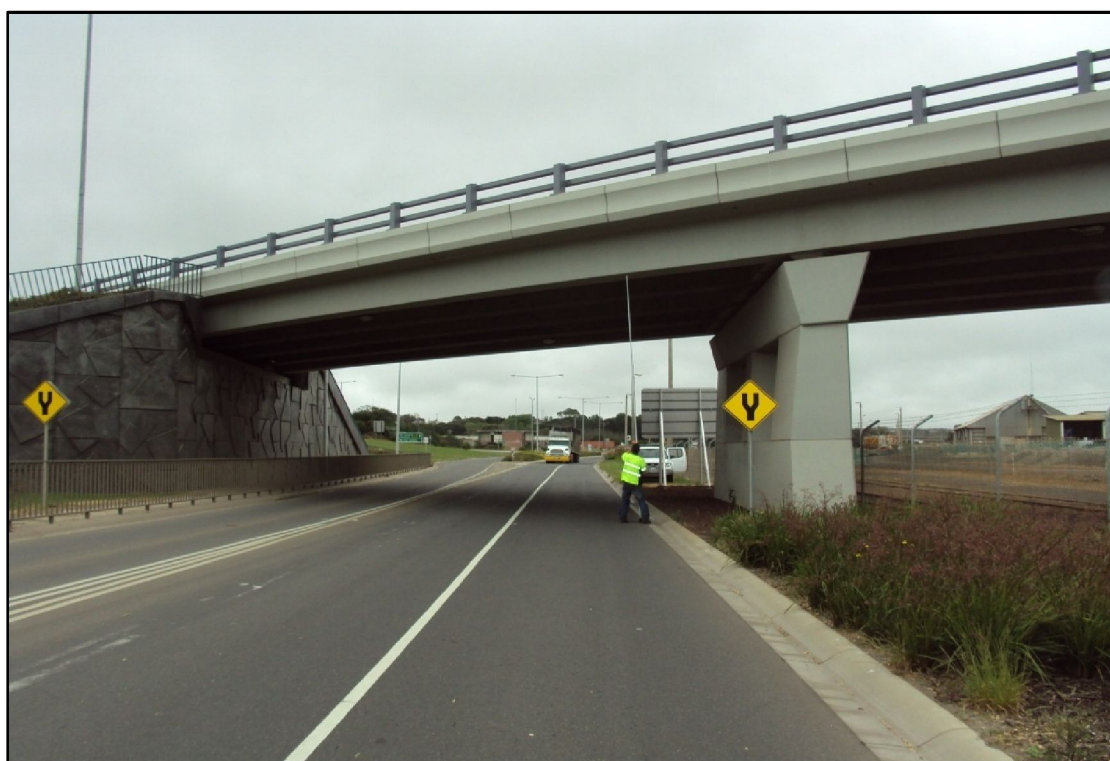
Figure 5.6: Identification of bridge underpass height risk
