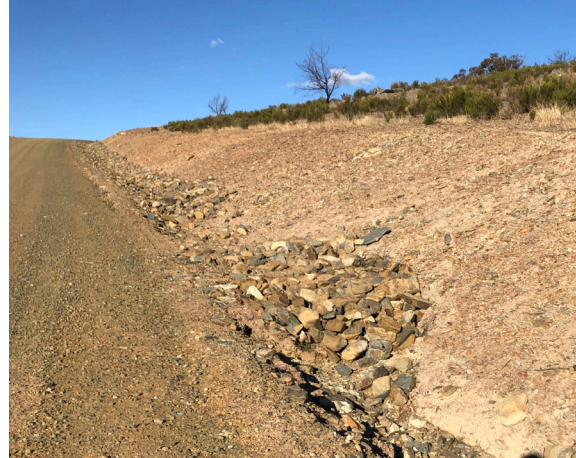
Figure 2 Rock Lined Drains
