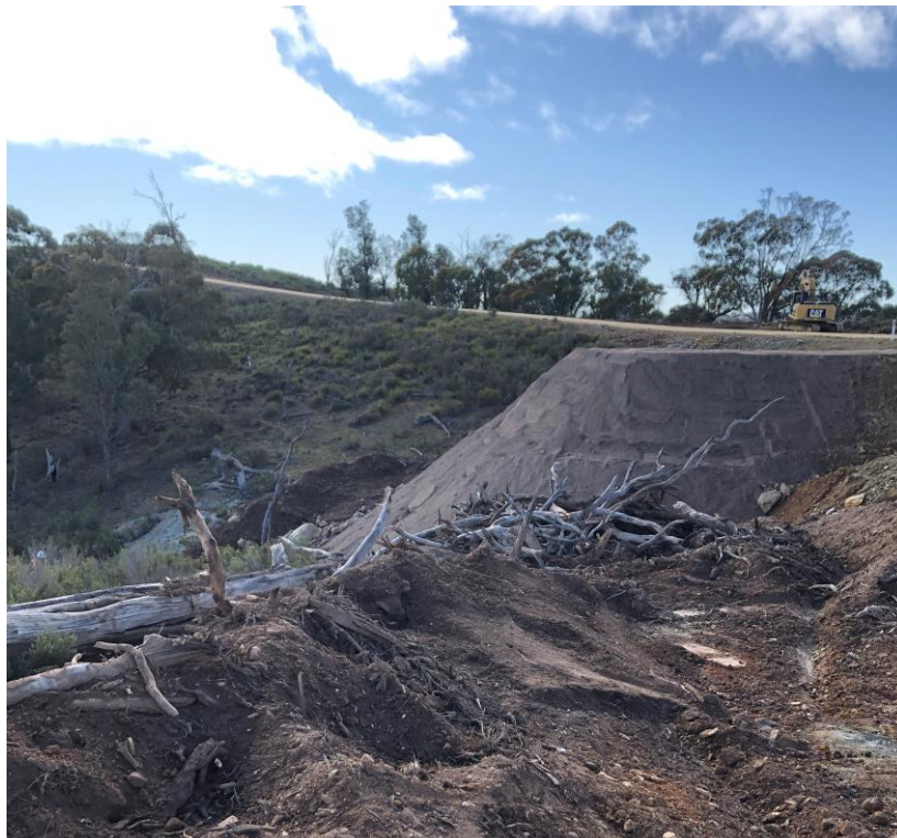
Figure 6 Unprotected fill embankments
