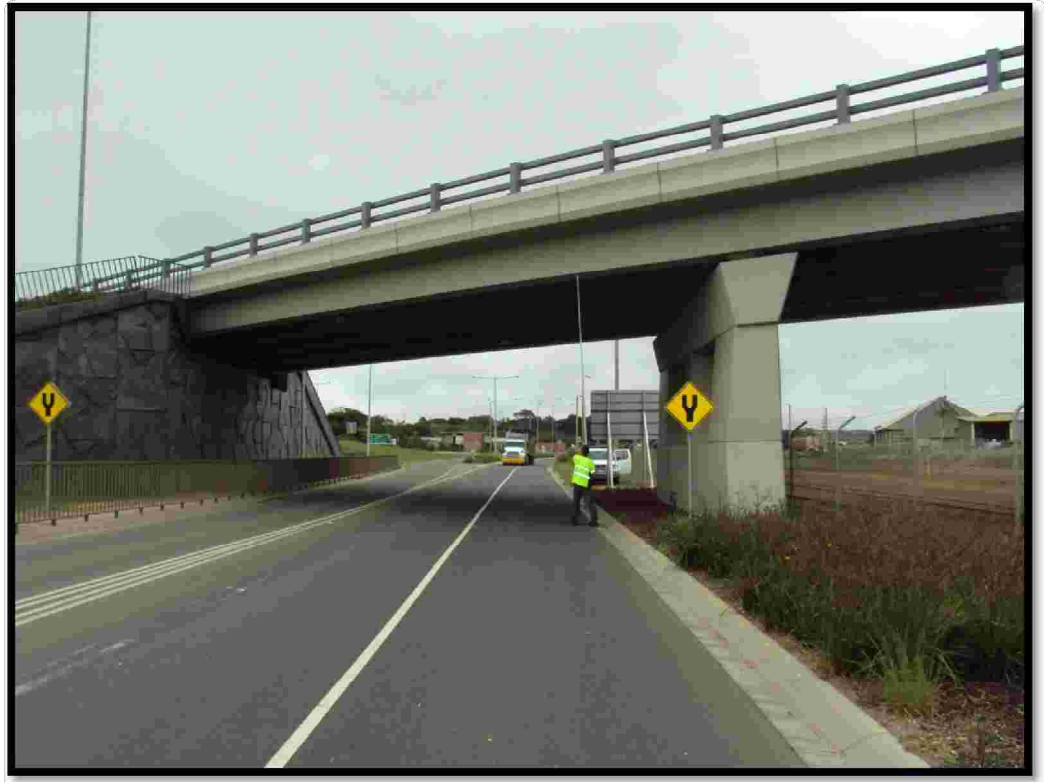
Figure 5.3: Identification of bridge underpass height risk
