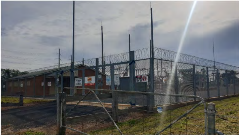
Plate 10: Looking northeast, electricity substation opposite subject site
