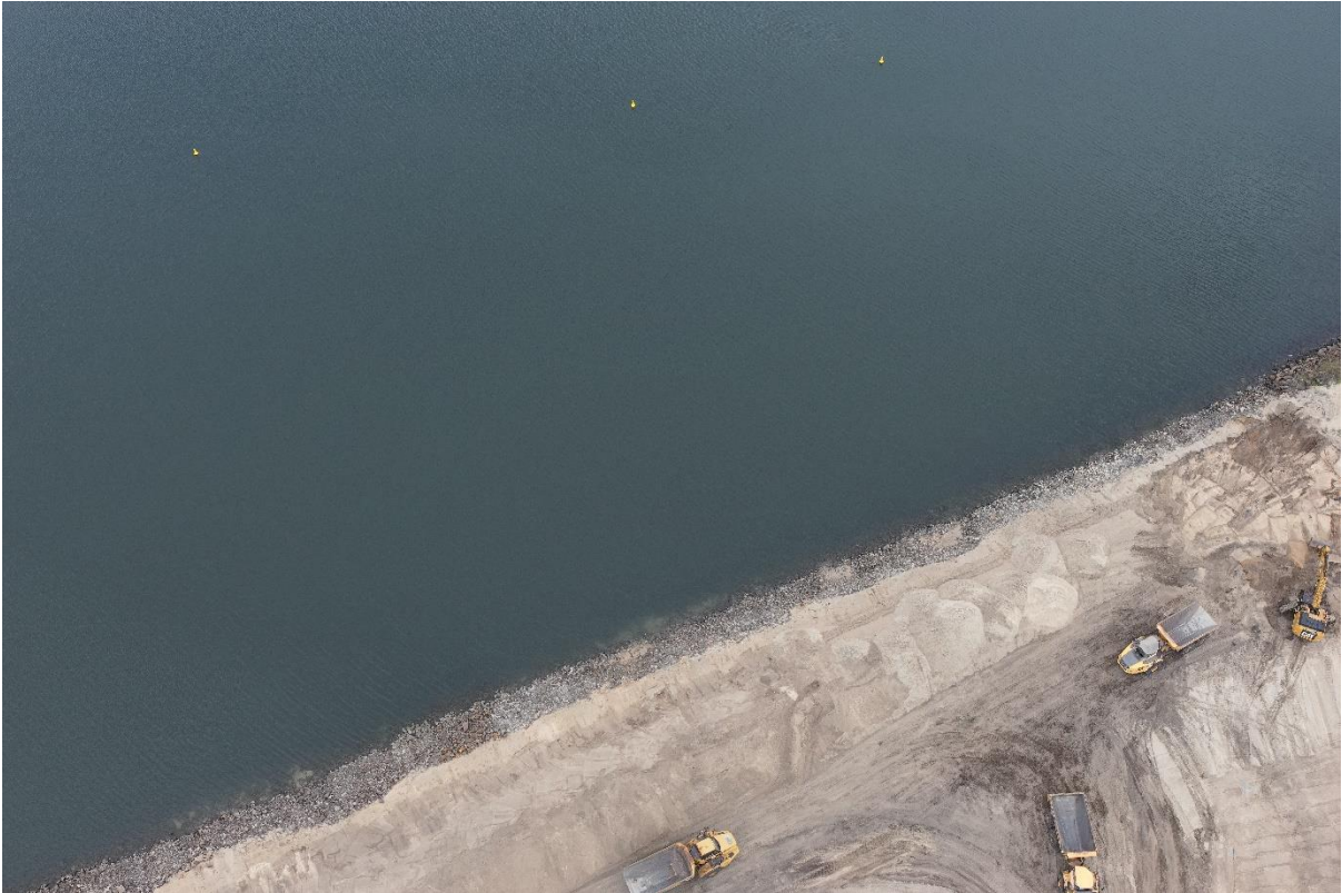
Photograph 1: View of removed wharf piles at Berth 101 and construction of piling pad for new wharf pile installation.
