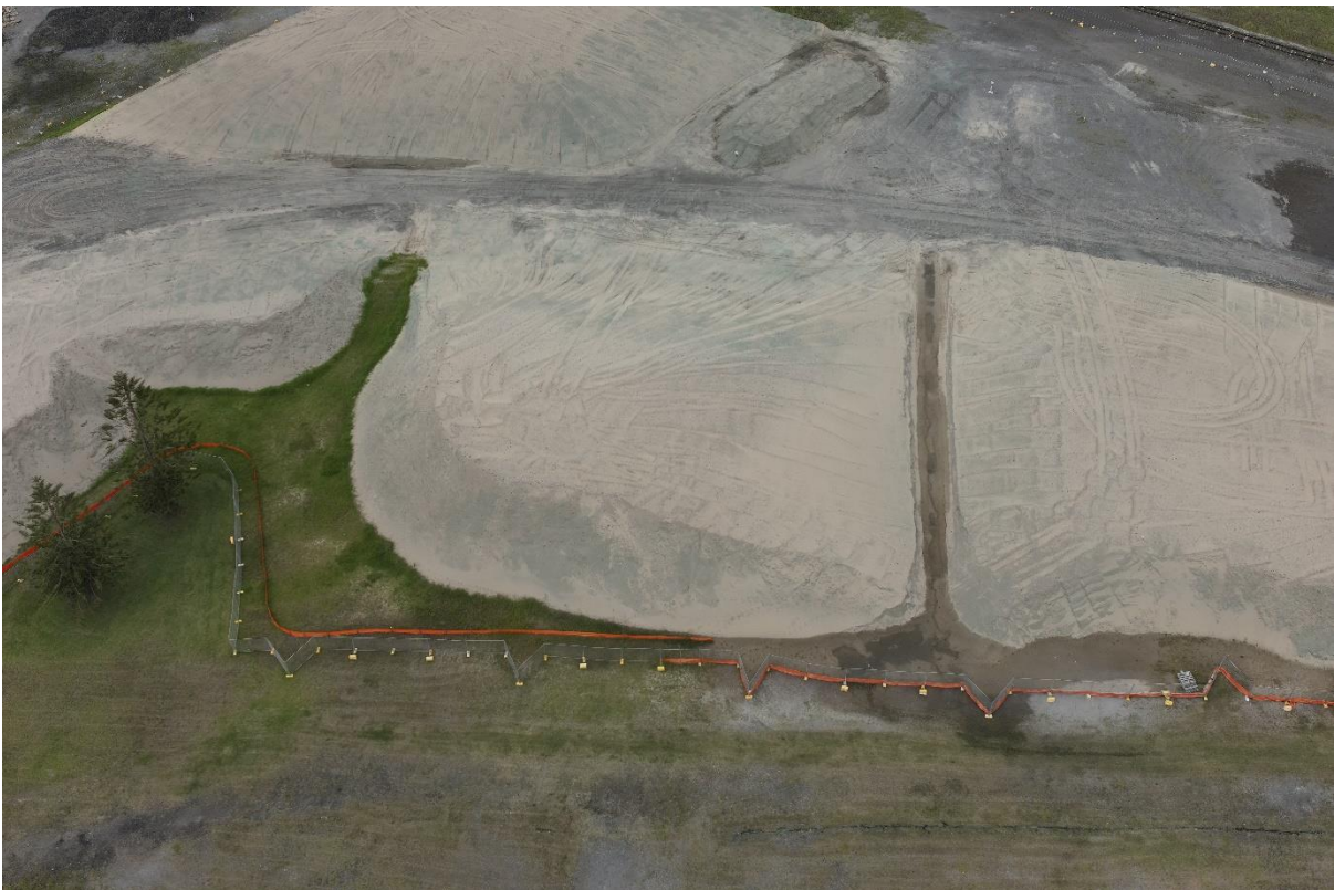
Photograph 2: View of Outer Harbour stockpiles showing polymer application and sediment controls in place.
