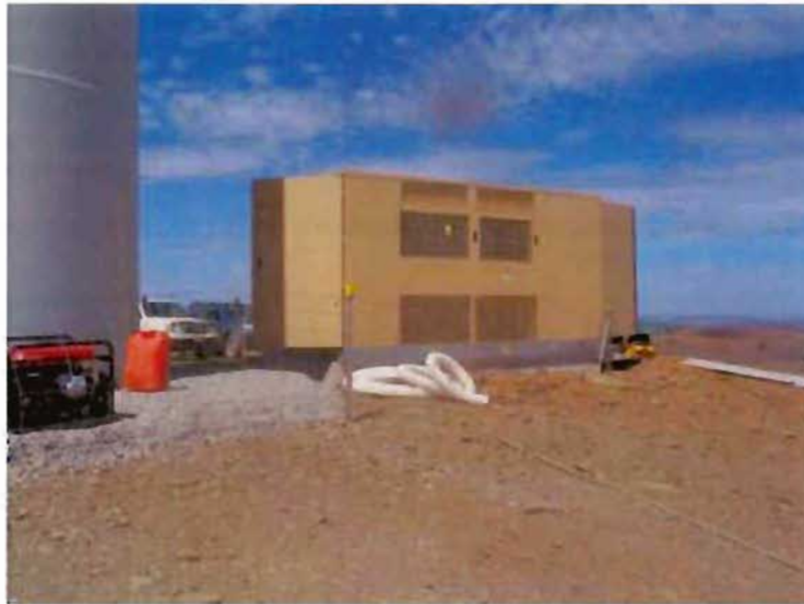
Image 5: Transformer adjacent to wind turbine
