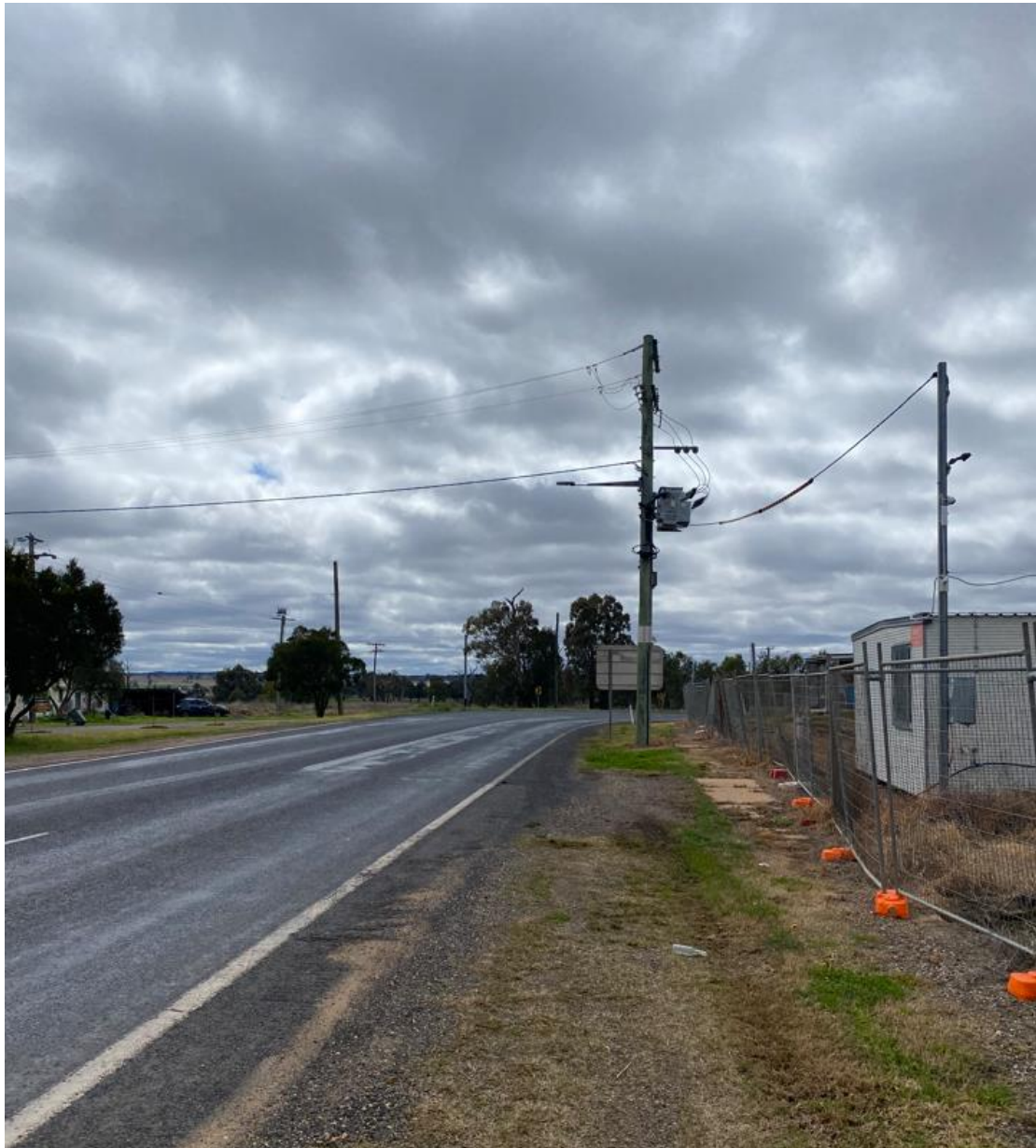
Figure 18 – Pole 39049 7084 (looking North)
