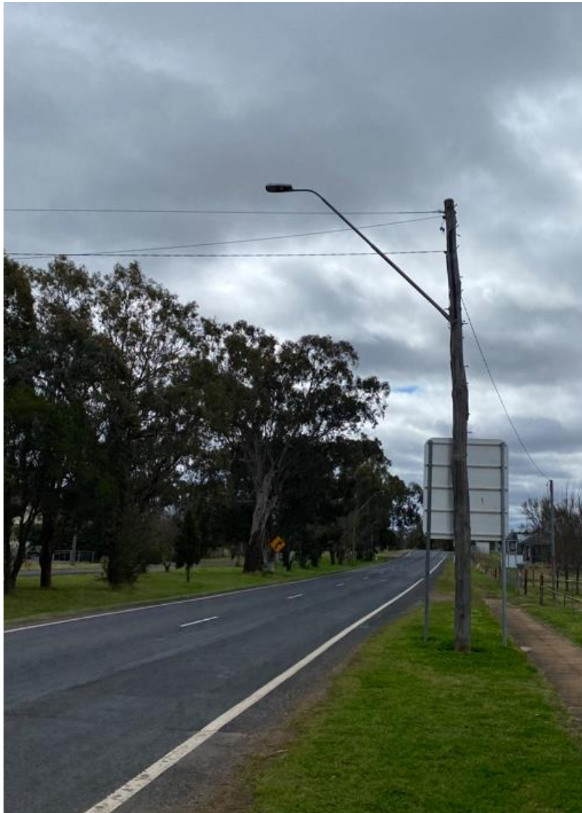
Figure 15 – Pole 39056 7084 (looking North)
